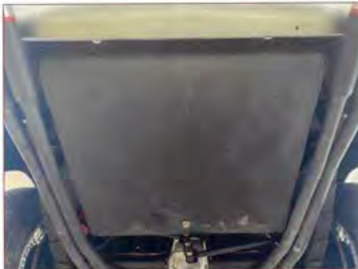
Serbatoio carburante (se accessibile) Fuel tank (if accessible)
